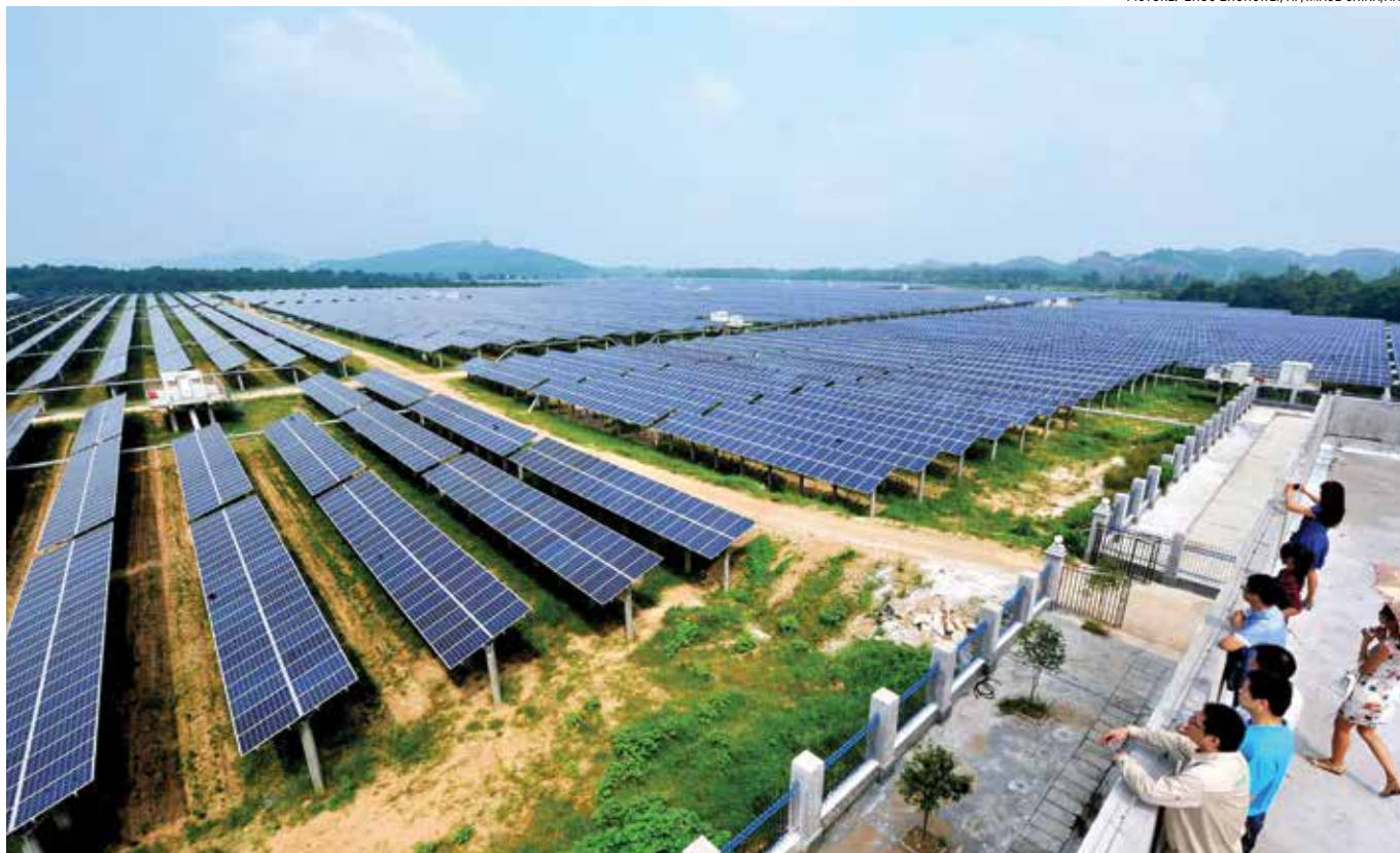
A photovoltaic power station in Heng Feng county of China's Jiangxi province in August 2015. The cost of solar power has fallen dramatically in China to be almost price-competitive with coal thanks to rapid technological advances.
