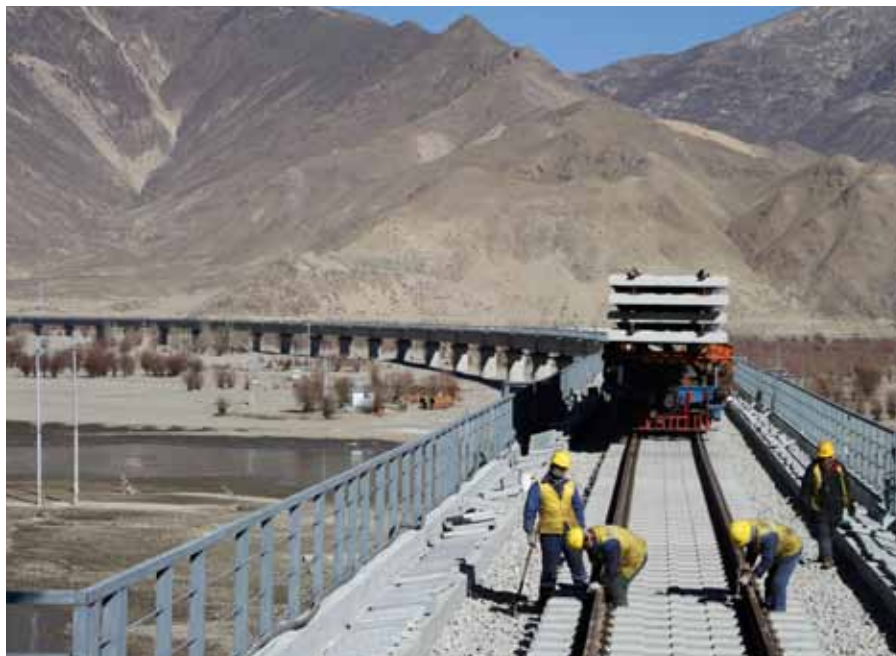
Workers fixing railway tracks on a bridge over the Yarlung Tsangpo river as part of the construction of the railway linking Lhasa and Nyingchi, Tibet. An international management council could balance needs and resource usage in the Great Himalayan Watershed.
