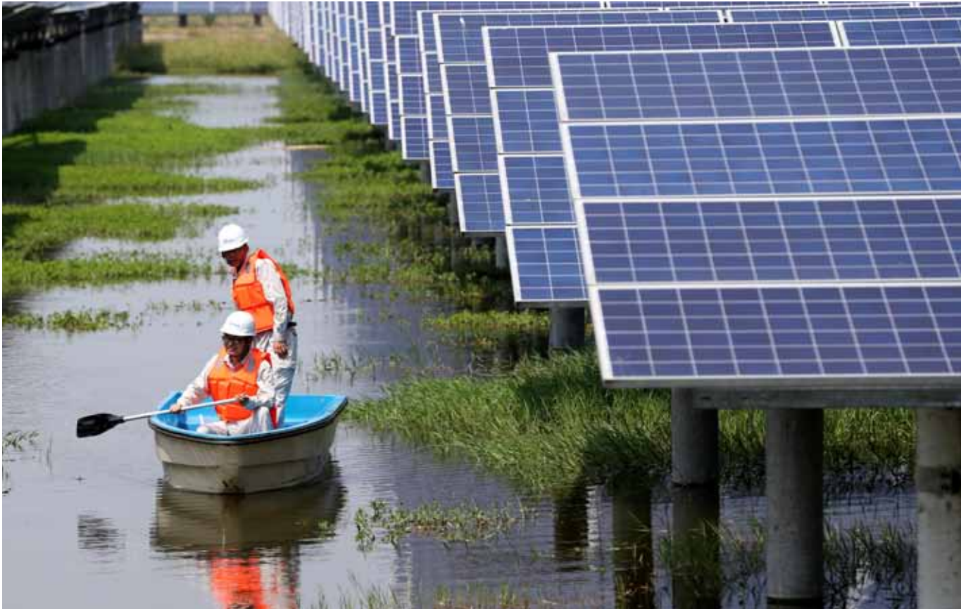
Employees check solar panels of a photovoltaic power generation project in Jingzhou, China. Energy in Asia will be 'profoundly shaped' by new technology.
