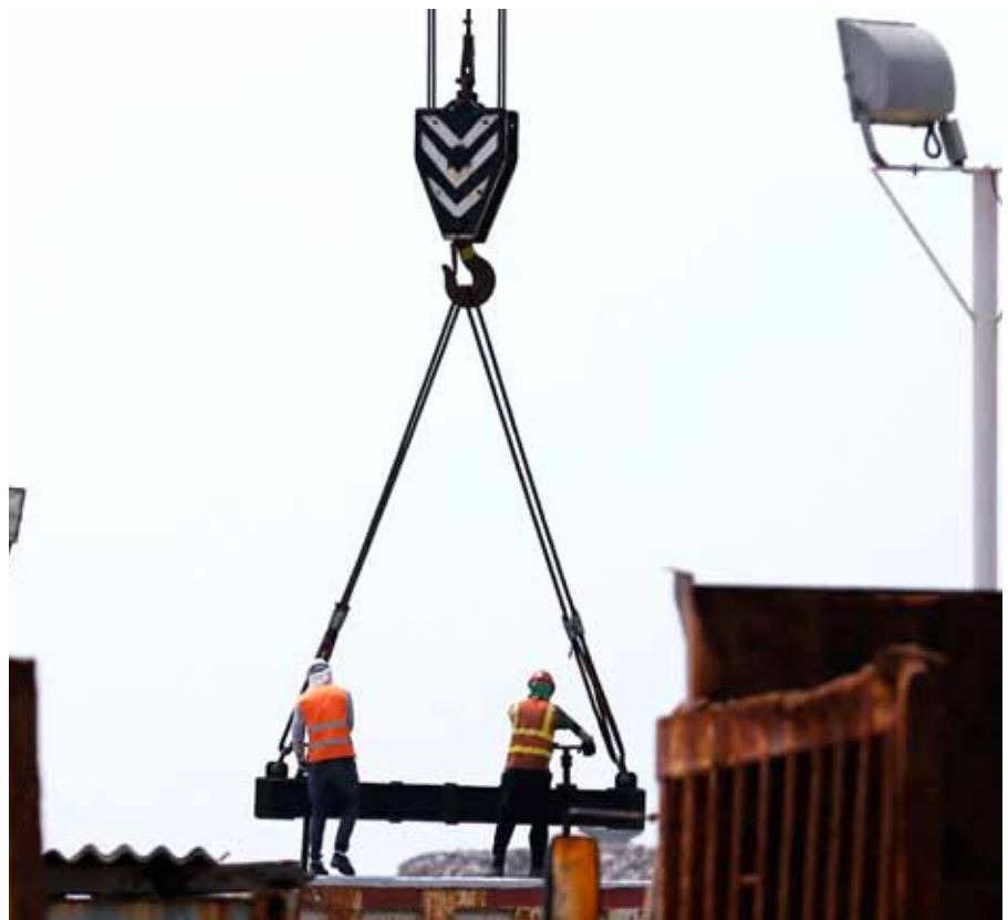
Men at work at the Colombo Port City, being built as an extension of Sri Lanka's commercial capital by a subsidiary of China Communications Construction Company Limited. President Xi Jinping has declared China's 'peace and development' strategy to be a fundamental foreign-policy goal.
